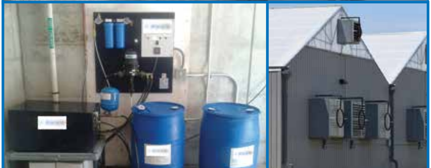
Installed FOGCO System
