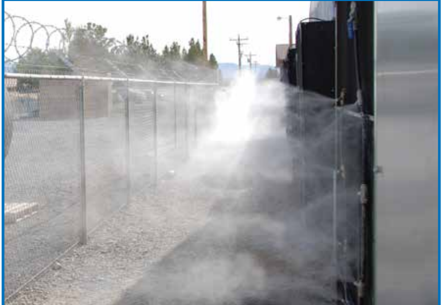
FOGCO System in Operation
